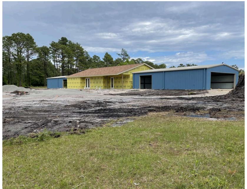
Roofs are up on the new clubhouse and cart barns, interior work is underway, and the new parking lot is taking shape.
